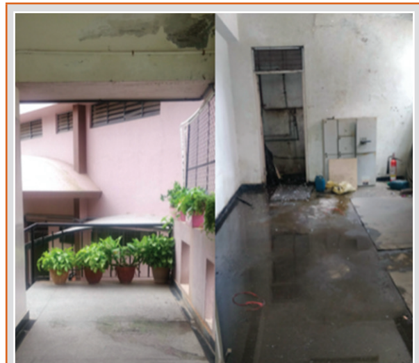
Figure 13 (b): Water collecting into a room with improper electrical fittings, right next to the school library.
